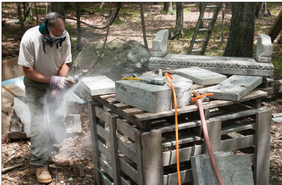
Michael Jamieson is in the middle of beveling and bush hammering newly fabricated stone components to match the antique bench shown in the background. He then carved hand and foot prints of his client's children into the surface of the seat. Most of Mike's work is done with smaller air and electric hand tools.
