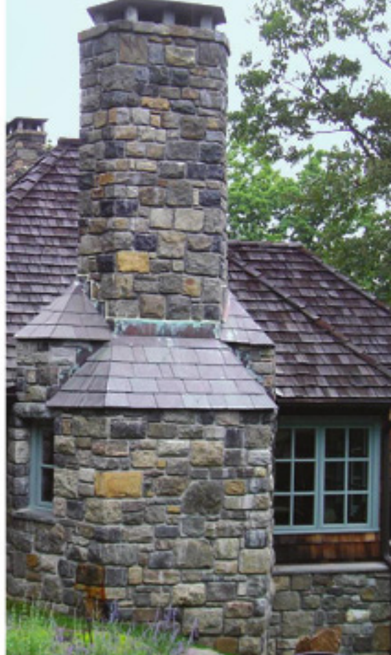
Lord Hillborn granite Chimney in Tuxedo Park, NY. Granite stone pier in Brooklyn, NY. Another set of entrance piers in Tuxedo Park, NY.
